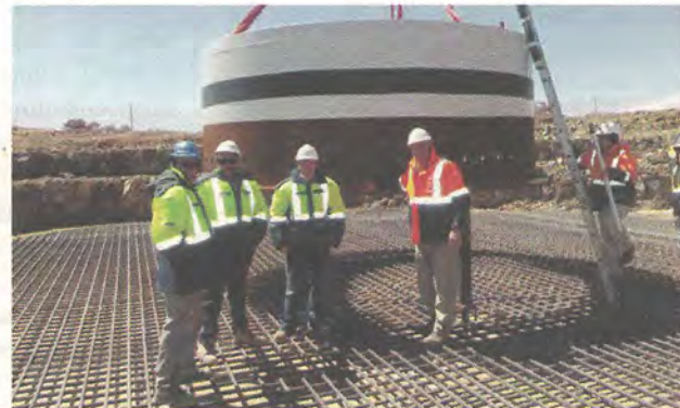
Above - The first of the tower embeds" being inserted into the foundation with Catcon employees and Origin's site manager in foreground.
