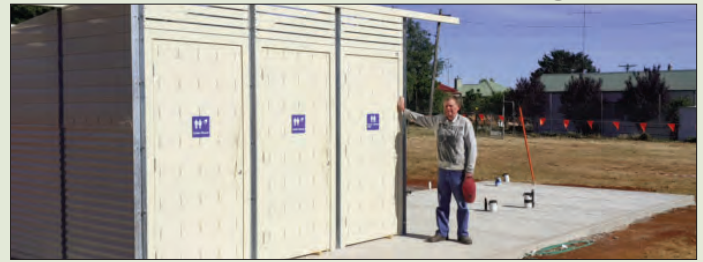
Crookwell Showground Committee President, Paul Anderson alongside the Toilet Block under construction at the Crookwell Showground. PHOTO: Linus Nesbitt-Hawes.
