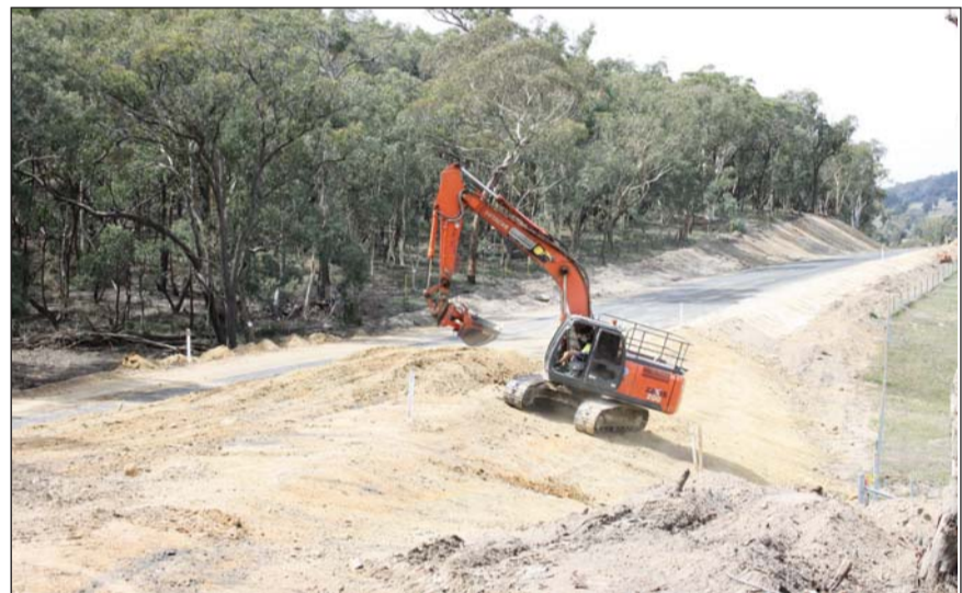
Right and Above: Works on the reconstruction of segment 475 near Junction Point Road Main Road 54.
