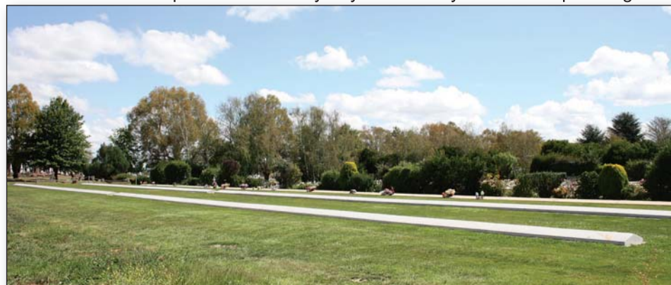
The newly constructed concrete plinths at Crookwell cemetery were completed by Council's outdoor works staff to increase the capacity of the cemetery and service community needs.
