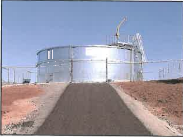
Water Storage Taralga Water Supply Upgrade
